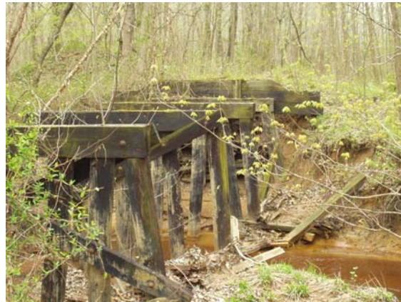
Remains of bridge near Madisonville
