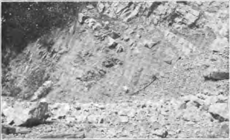
Plate 55. St. Louis limestone overlying New Providence formation. Quarry just south of Pineville, Ky. Looking northeast.
