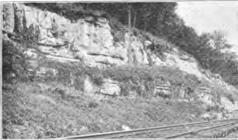
Plate 63. Natural exposure on Cincinnati Southern Railroad about one-half mile south of Burnside, Ky., showing Ste. Genevieve limestone above and St. Louis limestone below. Looking southwest. Contact at upper recess at base of massive bed. Nodules of black chert and Lithostrotion prolificum and L. canadense in the ten feet of limestone below recess.
