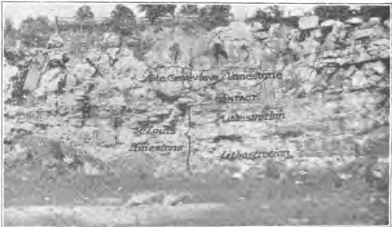
Plate 62. Old quarry one-half mile northwest of Somerset. Looking north. Ste. Genevieve limestone above, St. Louis below. Contact about middle. Layer with Lithostrotion proliferum six feet below contact.
