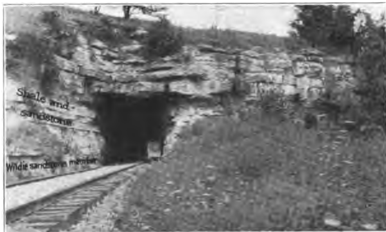
Plate 40. View of tunnel at Hummel on Knoxville branch, Louisville & Nashville Railroad, 4\frac{1}{2} miles northeast of Mt. Vernon. Wildie sandstone member of Warsaw at bottom and thick-bedded yellow Warsaw limestone at top. Looking north. Compare Plates 41, 42, and 46.
